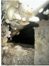
Hole in floor exposed.jpeg 1823K
