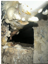
Hole in floor exposed.jpeg 1823K
