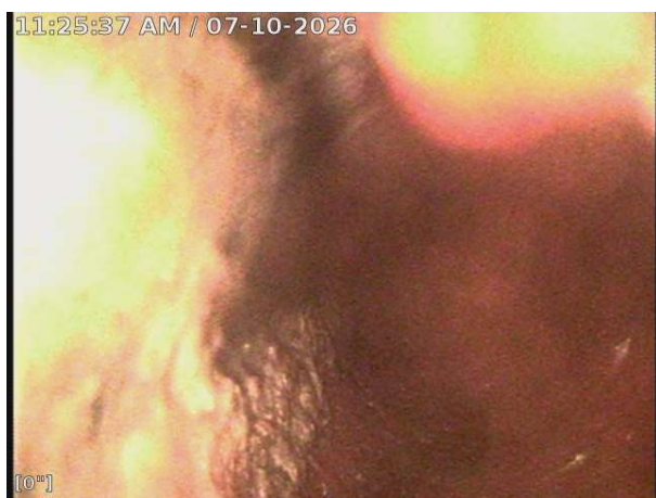
Start of cast iron sewer service pipe from cleanout in basement to sewer main in alleyway.
