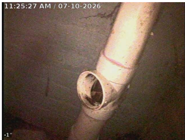
PVC cleanout in basement of 624 W. 33rd Street.
