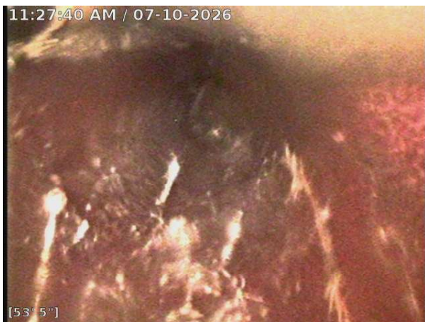
Root intrusion in sewer service pipe. This a potential future clogging point. This is located in the public right of way.
