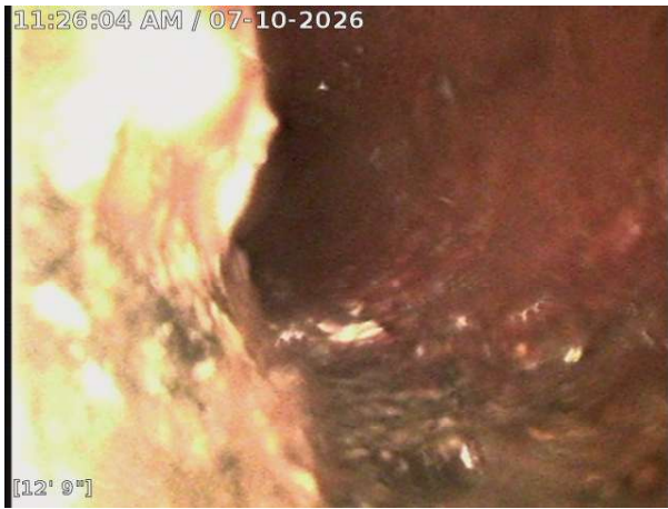
End of standing water in sewer service pipe.
