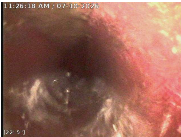
Change in pipe material from cast iron to terracotta.
