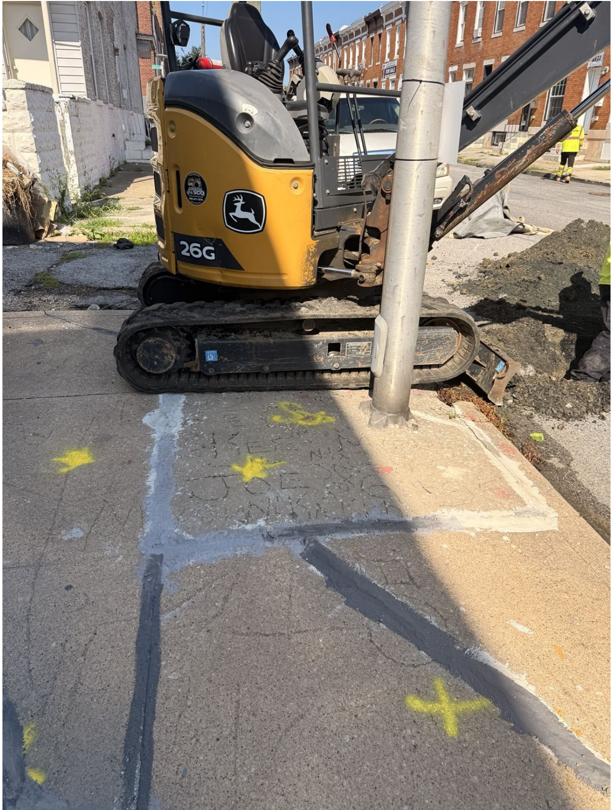
Photo 3 - Machinery positioned across the sidewalk beside visible cracking and patching.
