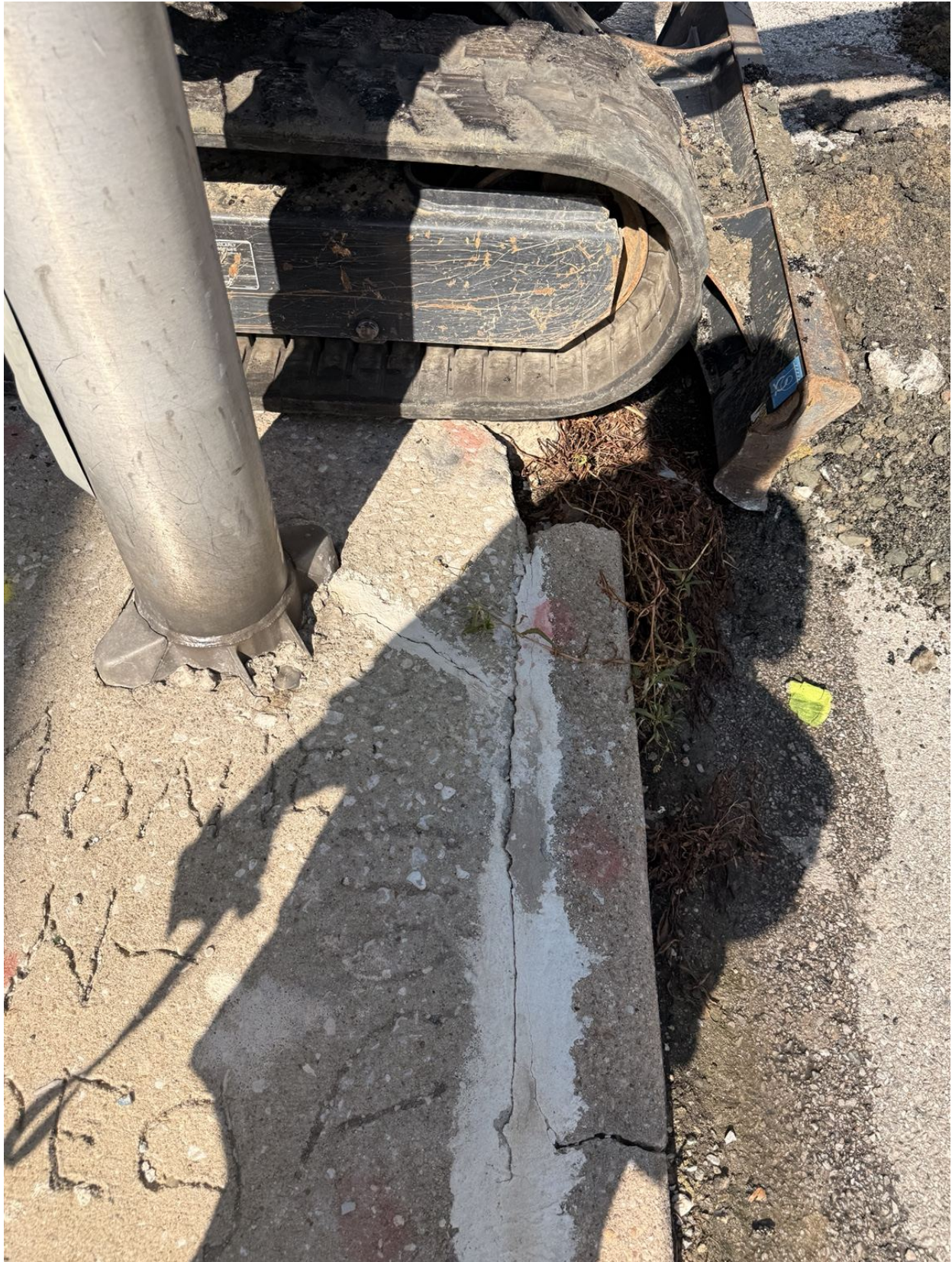
Photo 2 - Close-up showing the machinery track beside cracked and broken concrete.
