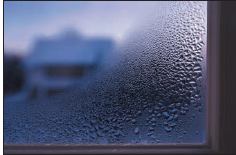
Condensation on the inside of a window-pane.
