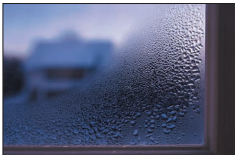
Condensation on the inside of a window-pane.
