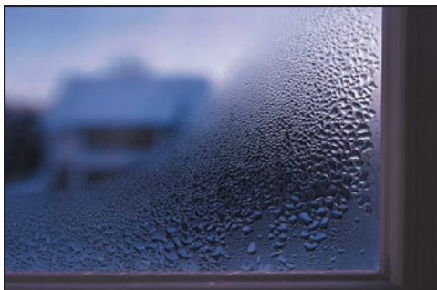
Condensation on the inside of a window-pane.
