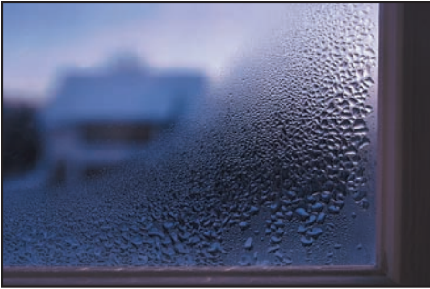
Condensation on the inside of a window-pane.
