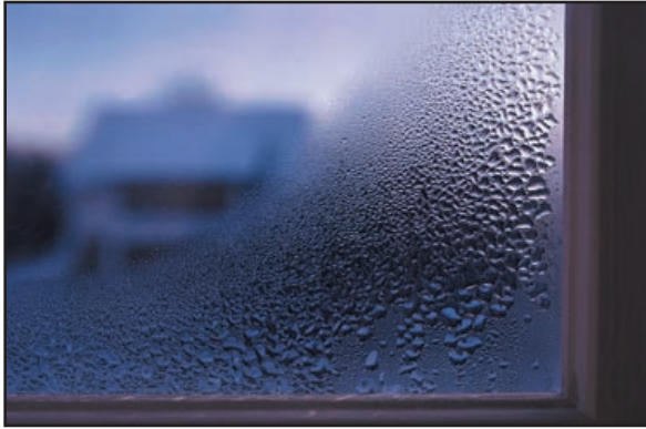
Condensation on the inside of a window-pane.
