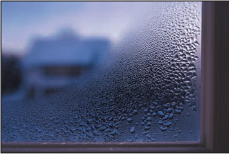
Condensation on the inside of a window-pane.
