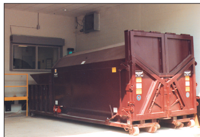
The DRC II meets the challenge of state requirements for waste and recyclables at this high-rise office building where space is limited. The covered installation provides additional convenience for personnel.
