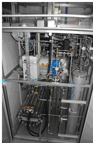
Fig 27.3(b) Small commercial electrolyser. Photograph courtesy of John Maddy, SERC, University of South Wales.
