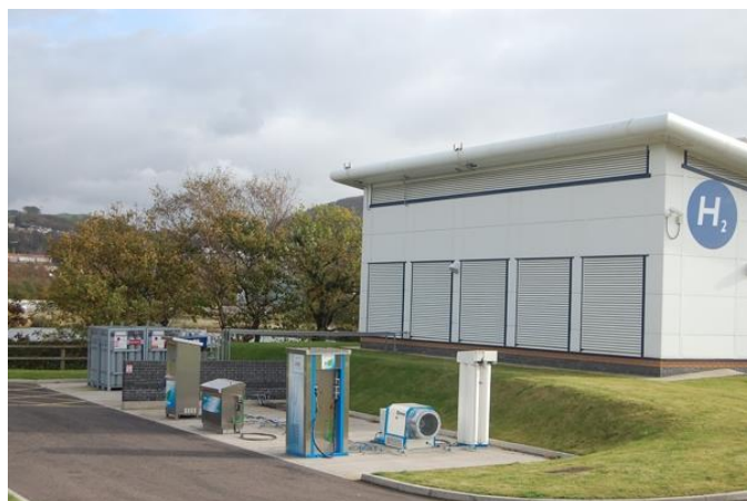
Fig. 27.2 Hydrogen vehicle refuelling area at Baglan Bay, South Wales. The building contains a commercial electrolyser which produces H_2 (see Fig. 25.3(b)) powered by photo-voltaic cells on the building roof. Photograph courtesy of John Maddy, SERC, University of South Wales.
