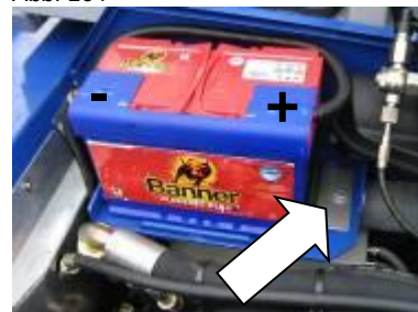
Position of battery 2
