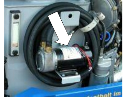
Hoses and fuel pump
