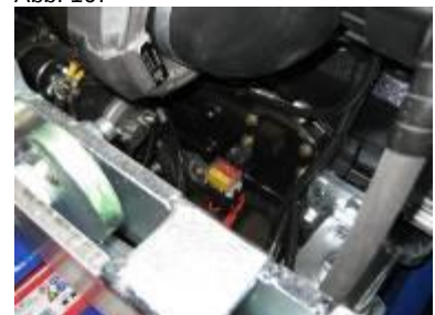
Location of fuse (engine room )
