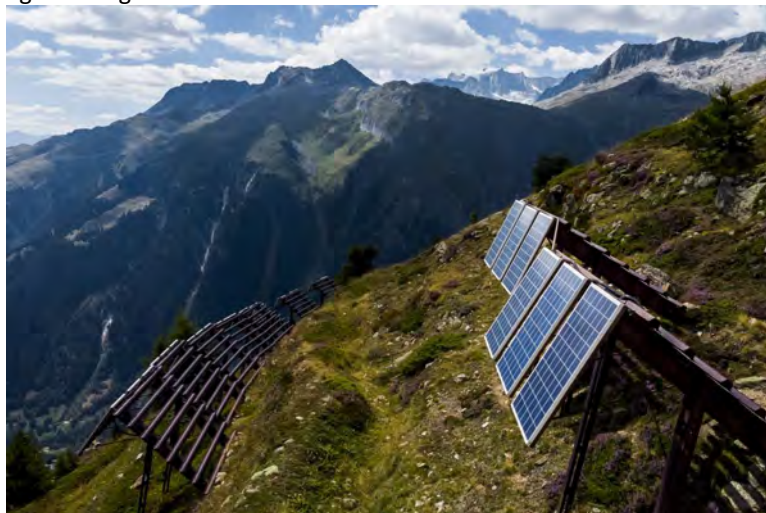
Figure 37 - Photovoltaic installation upon existing mountain infrastructure, such as avalanche protection (Keystone-SDA/RTS/sb, 2023), dams and road infrastructure.
