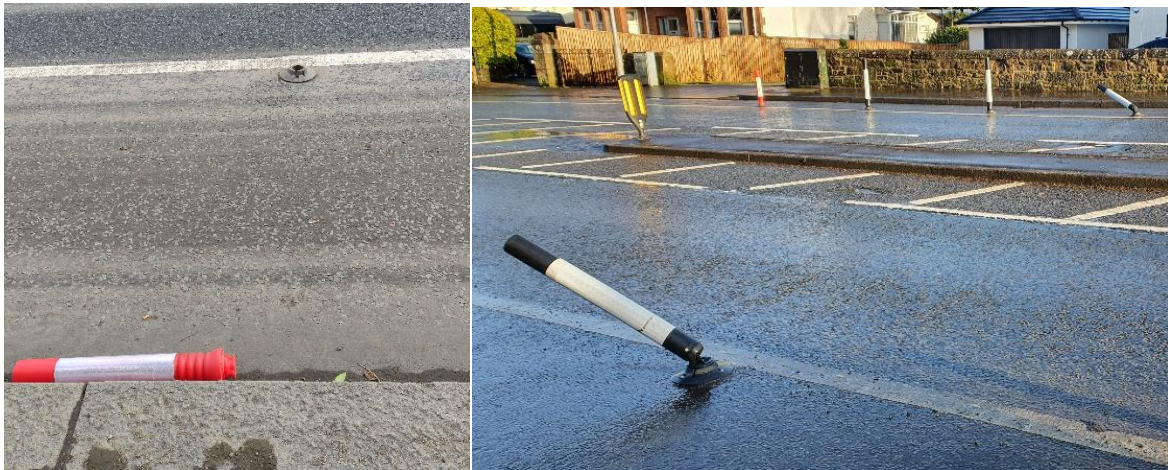
Fig 2: example of ongoing operational issues; bent, damaged and missing / dislodged bollards
