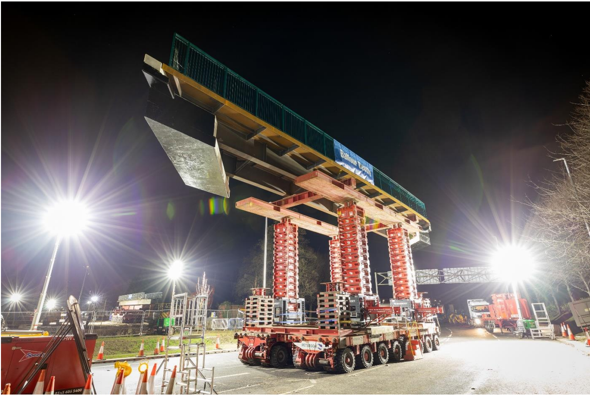
The new footbridge was transported using a special configured Self-Propelled Modular Transport (SPMT)
