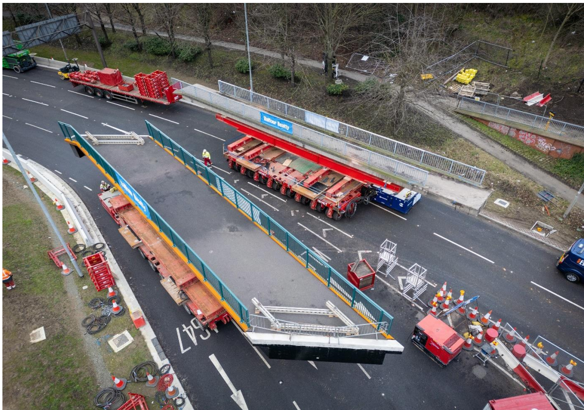
The new footbridge is more than twice the width of the old one.
