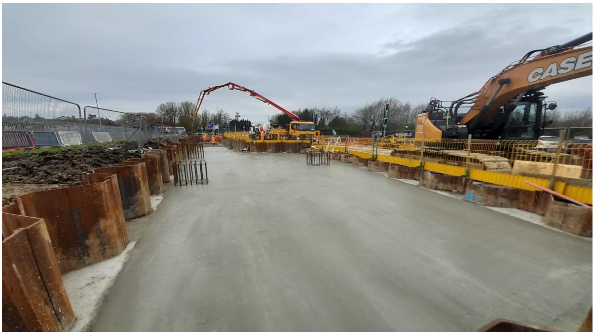
Phase two and three of the concrete pour for Spence Lane Footbridge
