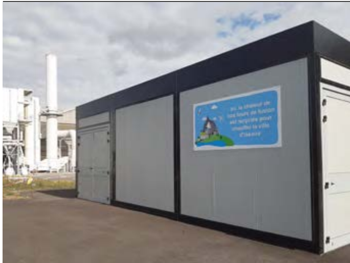
▲ This building contains the heat exchanger that provides heat to the city of Issoire
