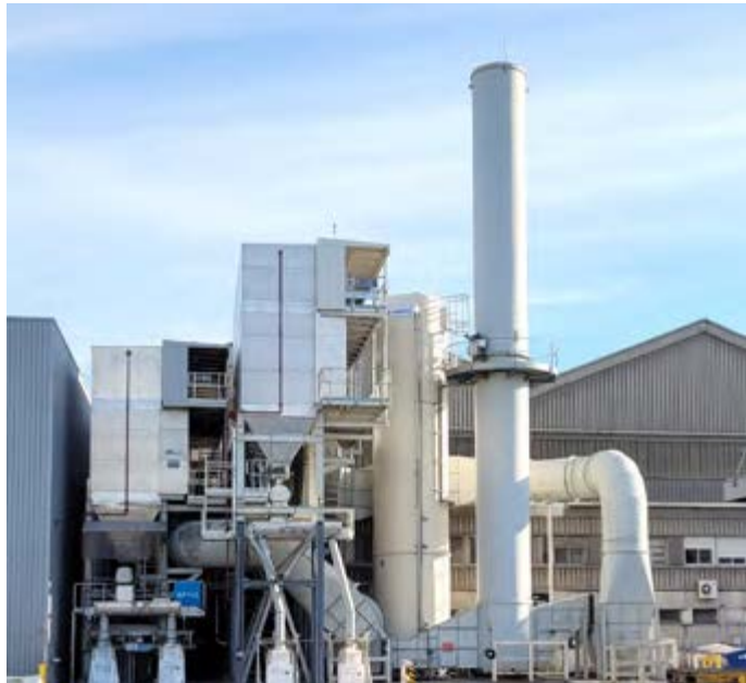
▲ Recently installed air filtering device at Issoire
