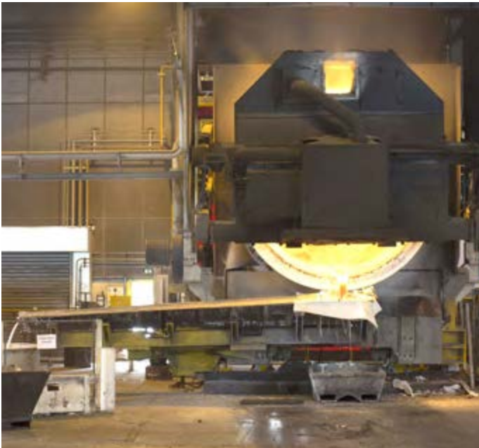
▲ Casthouse furnace at our site in Neuf-Brisach
