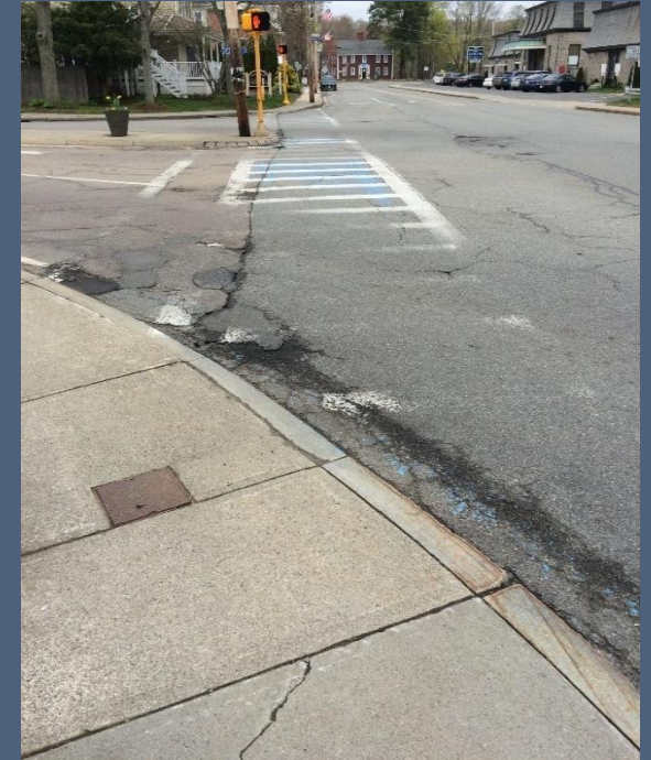
No Detectable Warning Panel
