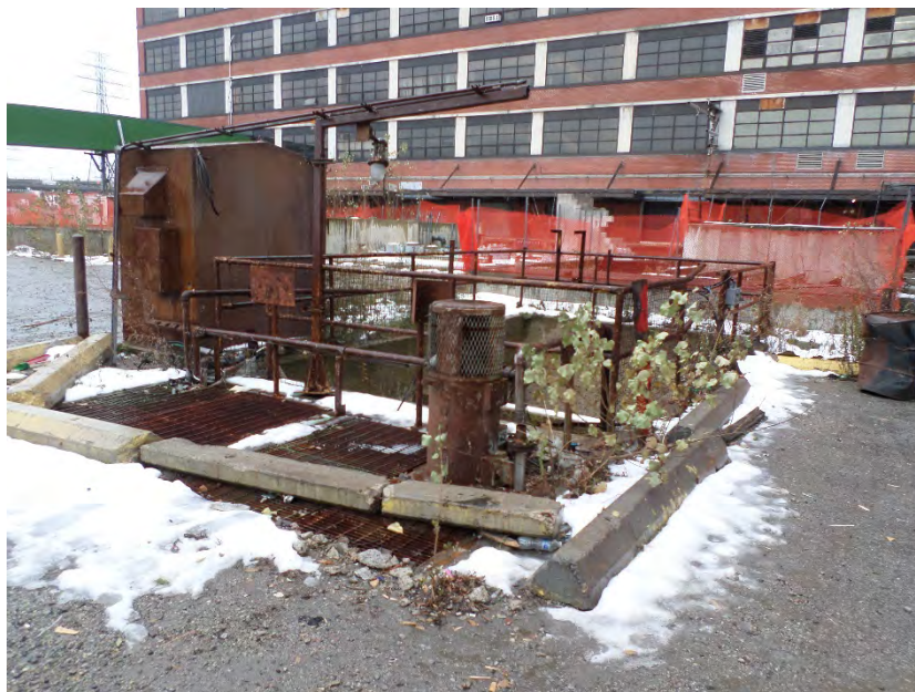
Photo 10 – View of former Pit #1 area and exterior tank areas located east of Building 36, facing southwest.
