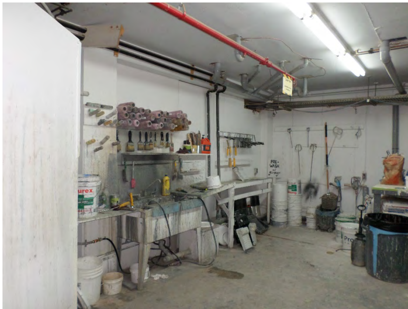
Photo 30 – View of paint storage room located within the building at 30 Booth Avenue.
