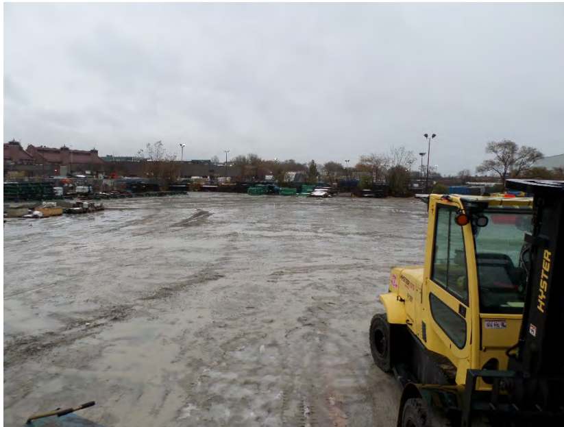
Photo 22 – View of the TTC leased work area located on the central portion of the Site, facing east.
