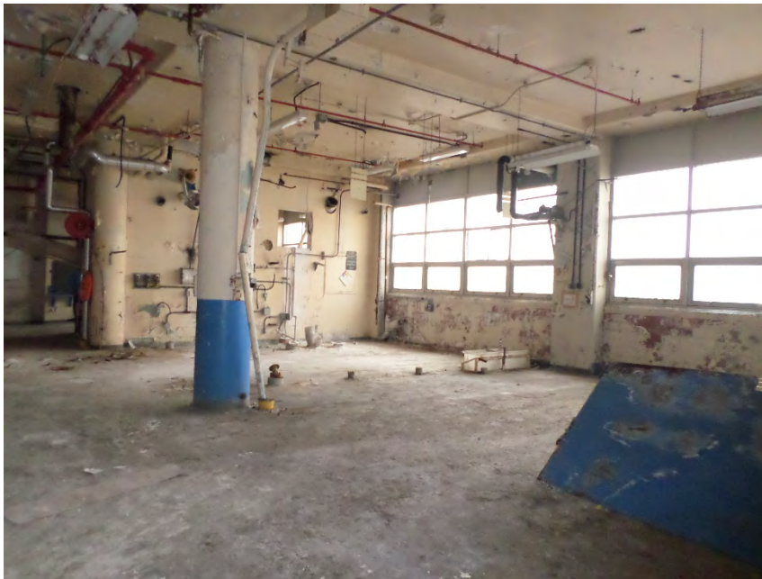
Photo 5 – Interior view of former manufacturing areas on the fifth floor of Building 36.
