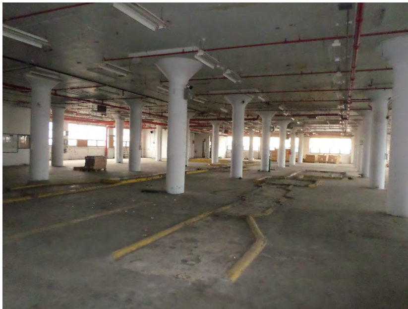
Photo 6 – Interior view of former manufacturing areas of the third floor of Building 36.
