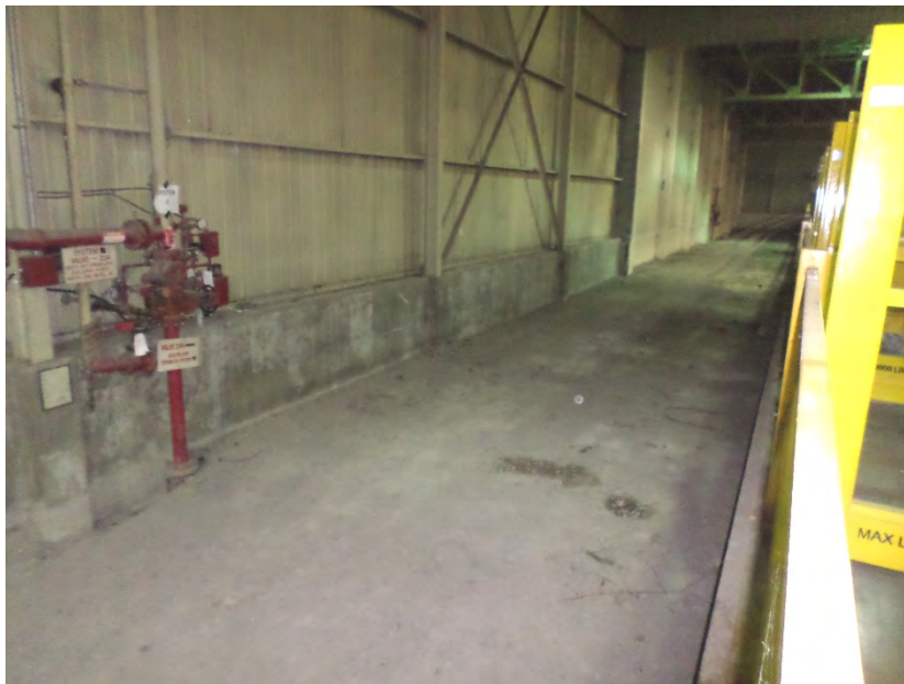
Photo 18 – View of former interior rail spur area, located in the southern portion of Building 41.
