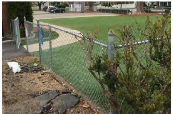
Accessible path connects to broken pavement
