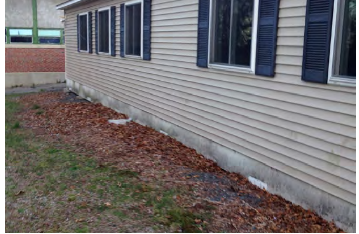
Signs of water damage along the base of the modulars
