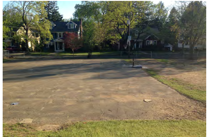
Cracking and uneven pavement
