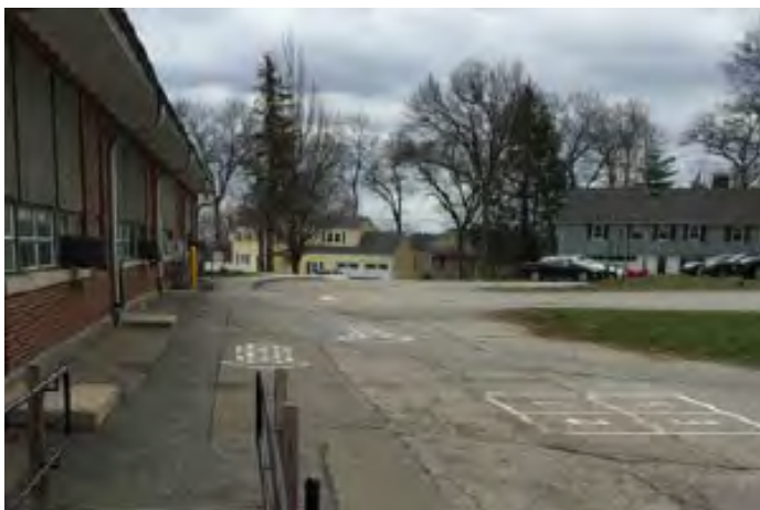
Pavement games on cracked asphalt by drop-off
