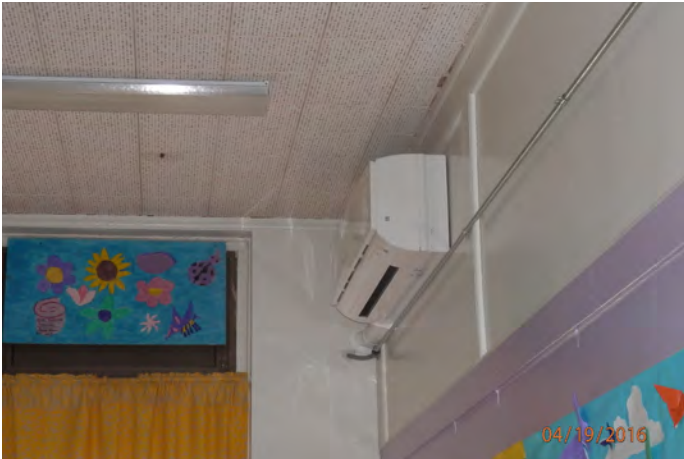
Recently installed air conditioning unit
