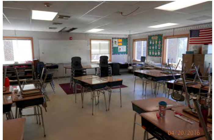
Typical lighting in classrooms
