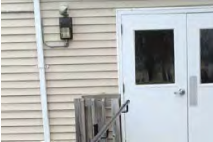
Lighting at modular classrooms
