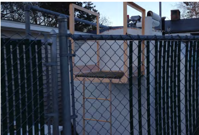
Steel oil tank adjacent to modulars
