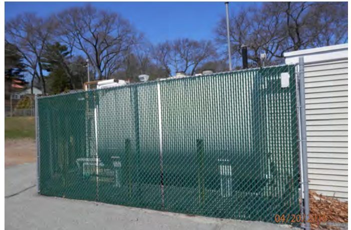
Generator for modular classrooms
