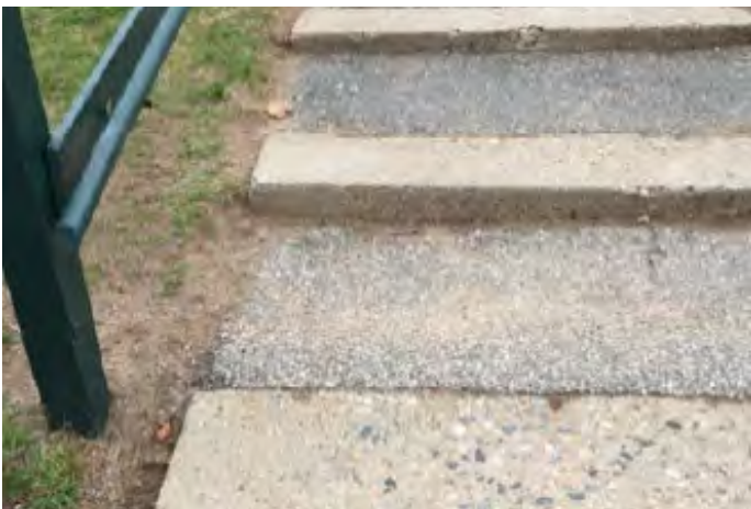
Worn condition of steps
