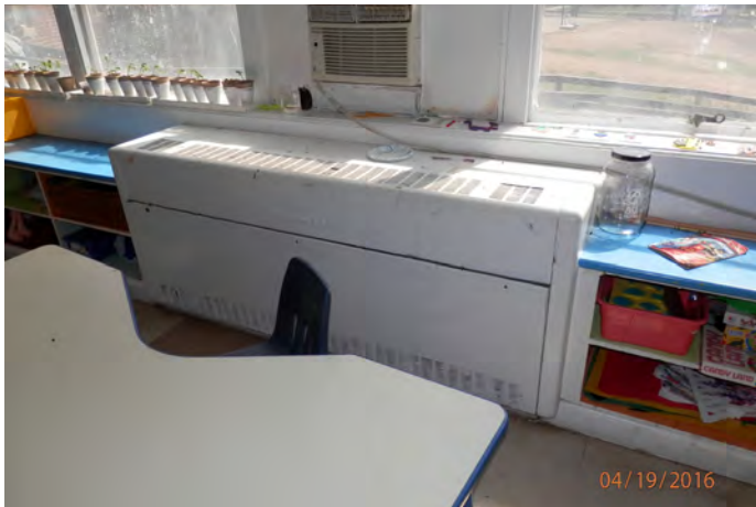
Typical heating system in classroom
