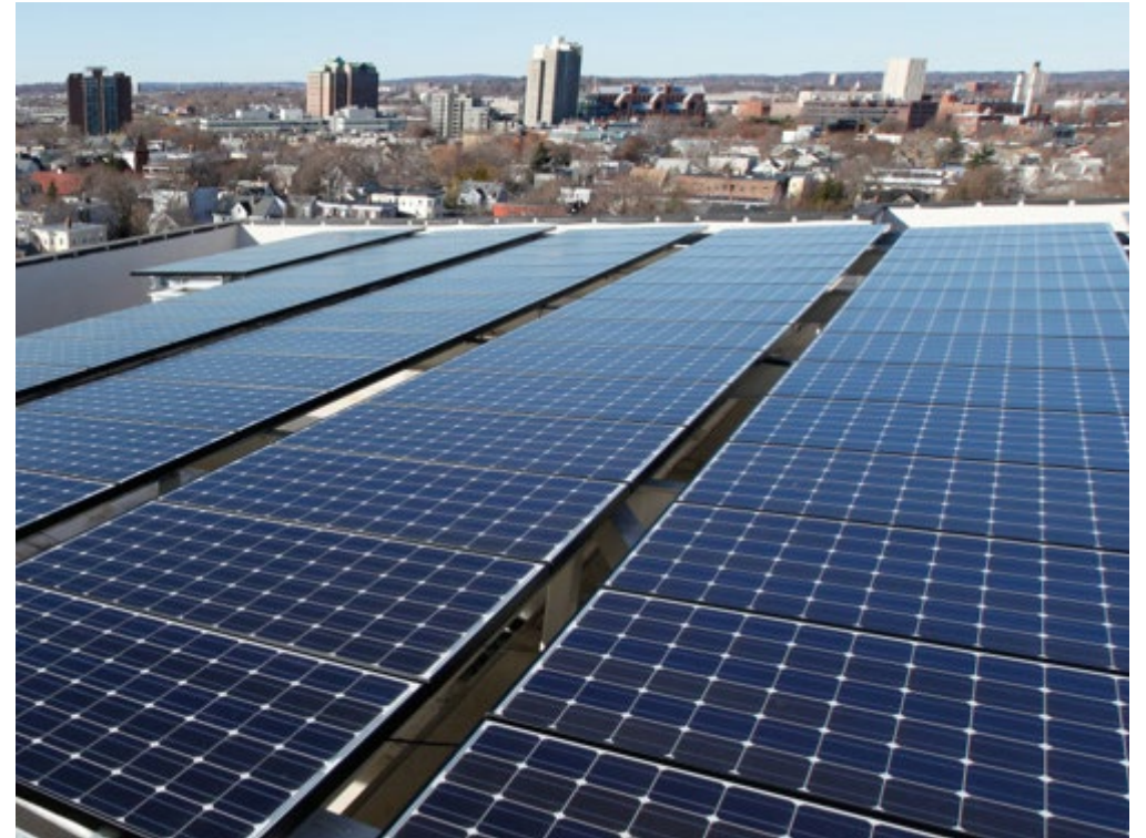
CHA's solar array at LBJ Apartments in Cambridgeport
