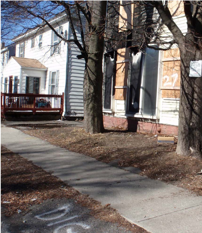
Boarded up residential structure on Orchard Street
