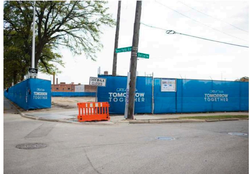
Expanded Sidewalk on Rosa Park Boulevard as Part of the Brass Factory Demolition.
