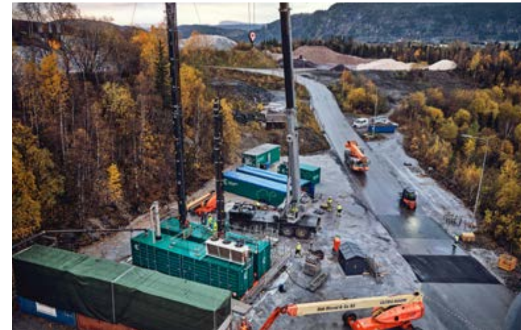
Credit: Brevik Heidelberg Capture Plant, image courtesy of Aker Carbon Capture
