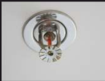
SMOKE DETECTORS AND HEAT DETECTORS
