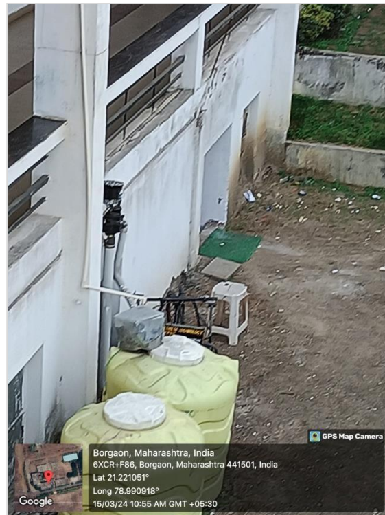
Plate 1: Rain water harvesting tanks in the premises
