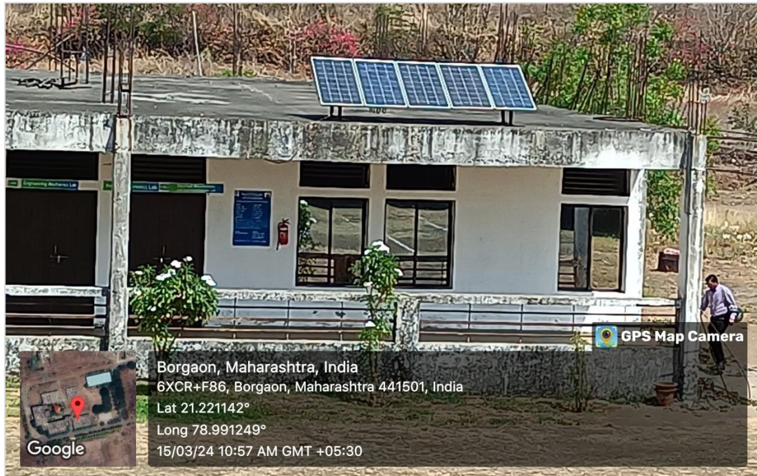
Plate 1: Rooftop solar panels in the premises
