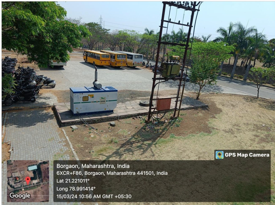
Plate 3: Main electricity generation areas in the premises
