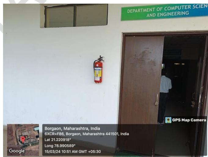
Plate 4: Fire extinguisher in the premises
