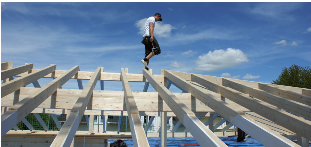
Joiner on the roof frame of the well-being bungalow with Feng Shui
