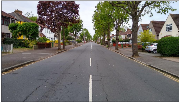
Infrastructure giving up at a junction.
