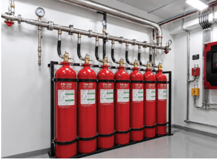
FM200 Fire Suppression System
