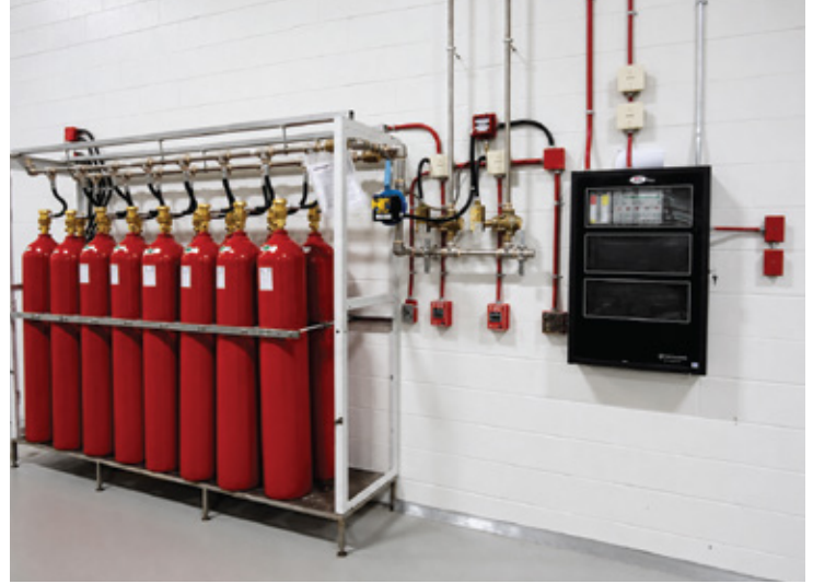
CO 2 Fire Suppression System
