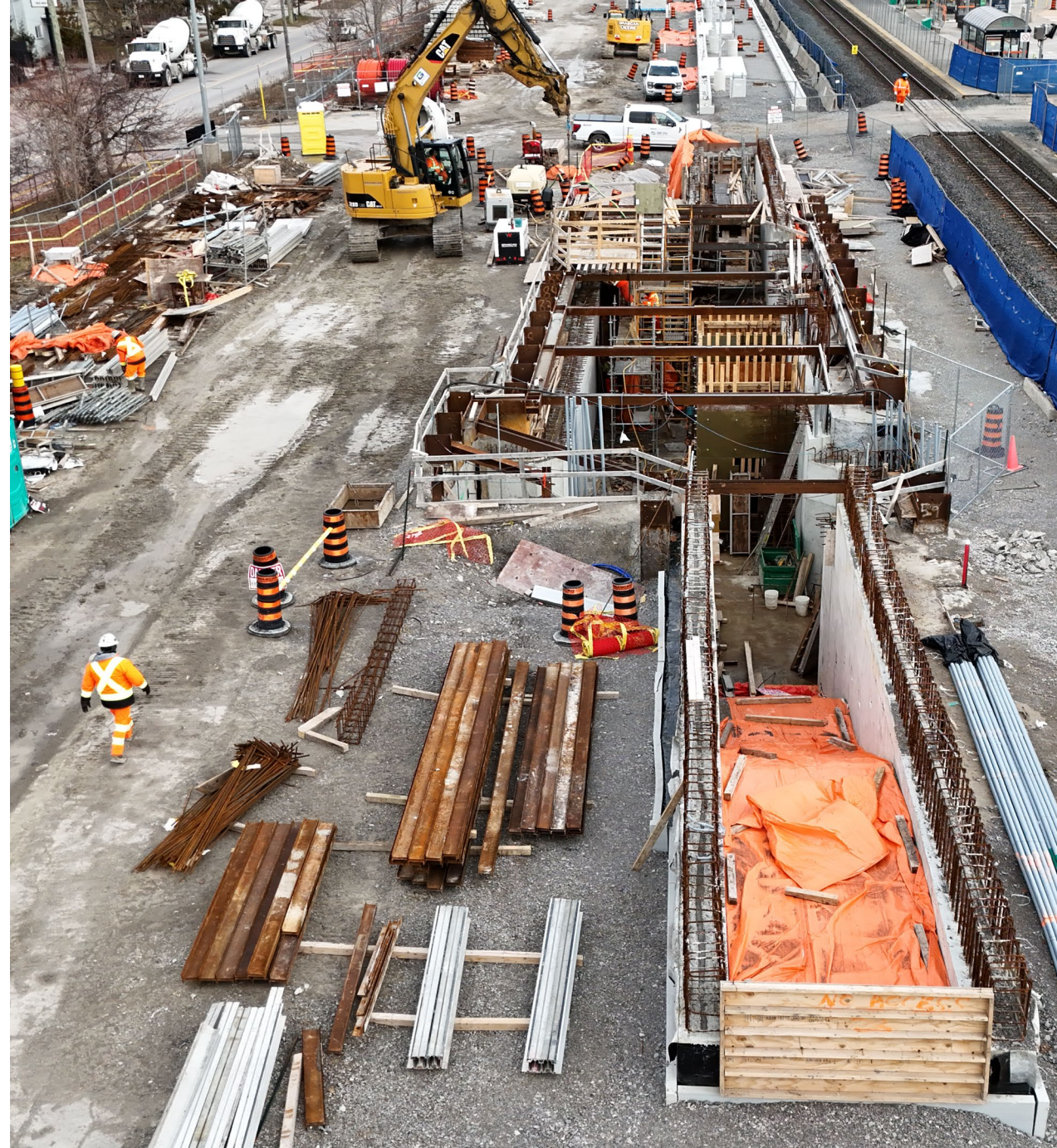
Forming and form stripping work as part of west tunnel construction activities. Metrolinx Image
