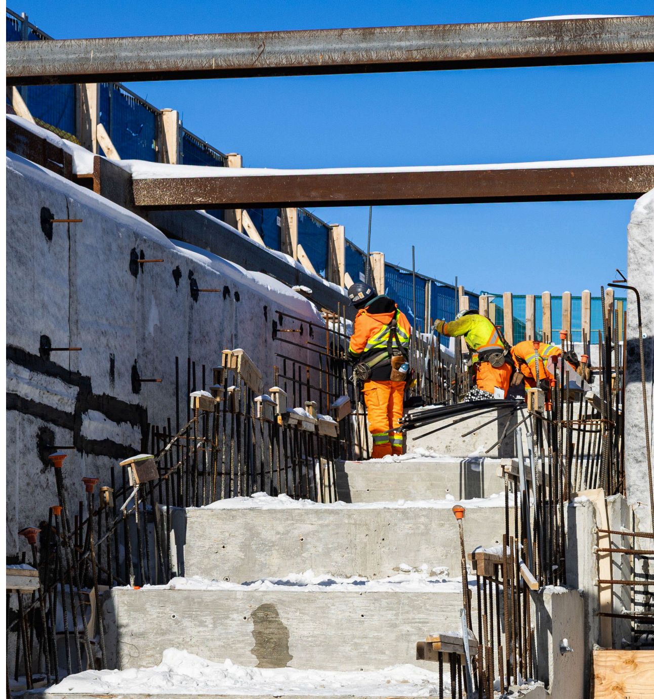
Site workers tying rebar on the north staircase walls of the east tunnel. Metrolinx image
