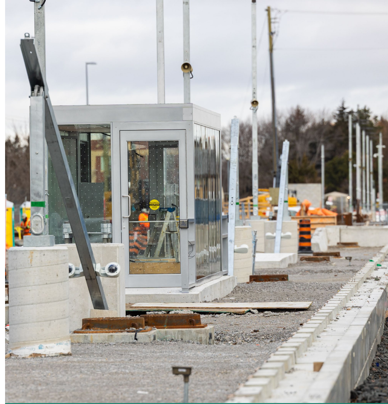
Works in the west platform area, including the shelter structure, utility and light poles, and electrical handwells for power and communication conduits. Metrolinx image
