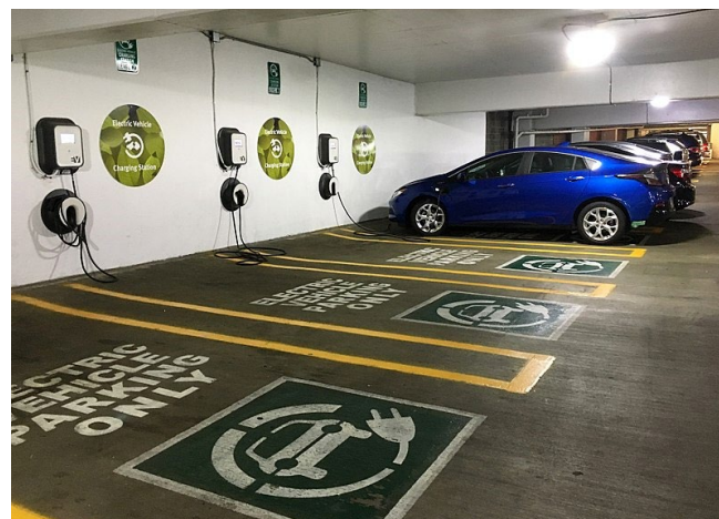
5 contiguous spaces adjacent to an electrical room are typical in parking garages
