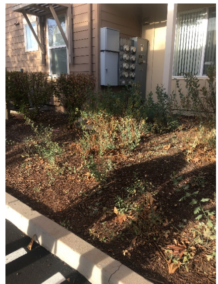
Short trenching distance with no concrete between house panel and parking spaces.
