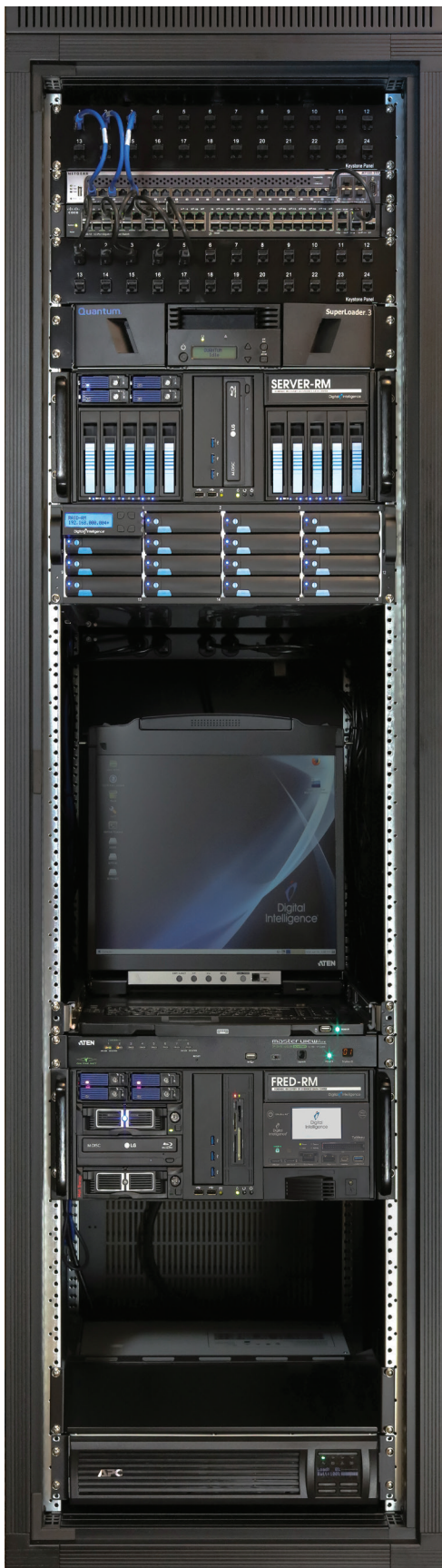
FREDC showing (from top): network switches, tape subsystem, Server-RM, RAID-RM™, monitor and keyboard, KVM switch, FRED-RM™ and UPS
