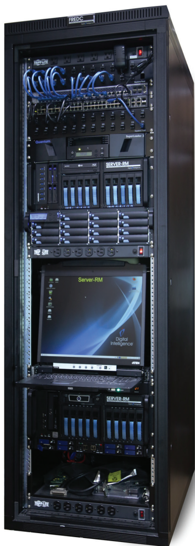
FREDC™ Data Center
