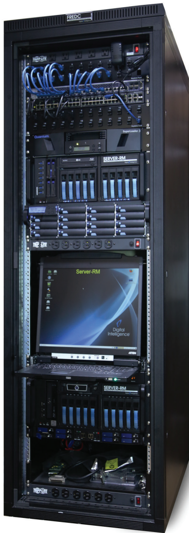
FREDC Data Center
