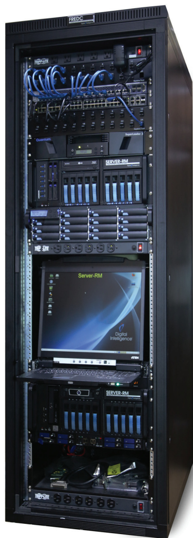
FREDC Data Center
