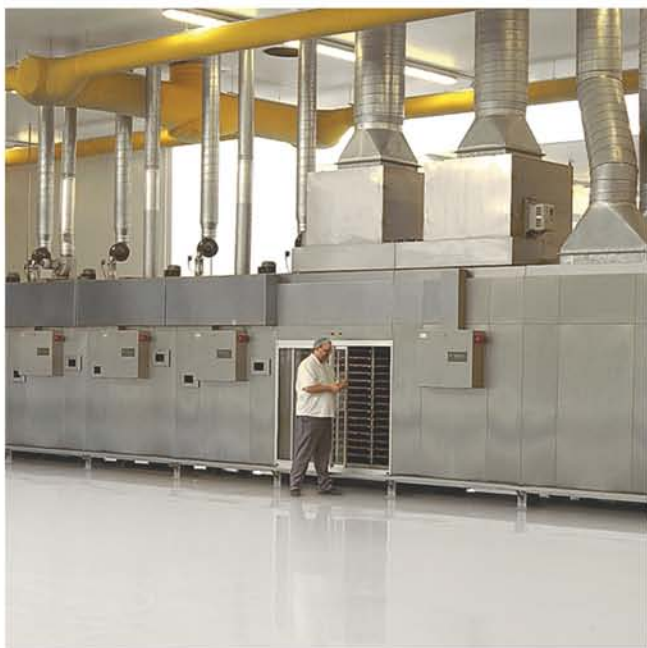
Picture: two cooler modules with inspection
