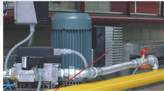
inverter for air speed control, mounted on motor
