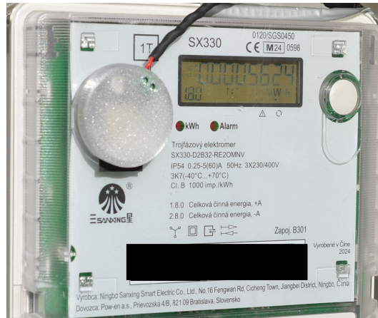
Picture 3. WOH-01 mounted on Energy meter
