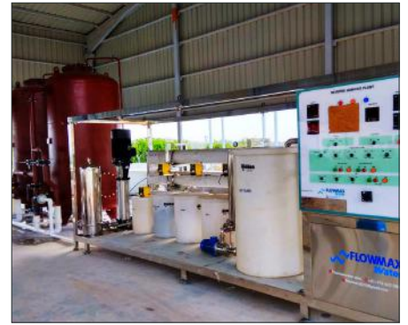
Fully automated RO plant- AVT, Tiptur - Karnataka
