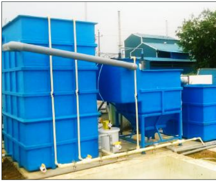
STP with MBBR technology - AVT, Tiptur - Karnataka
