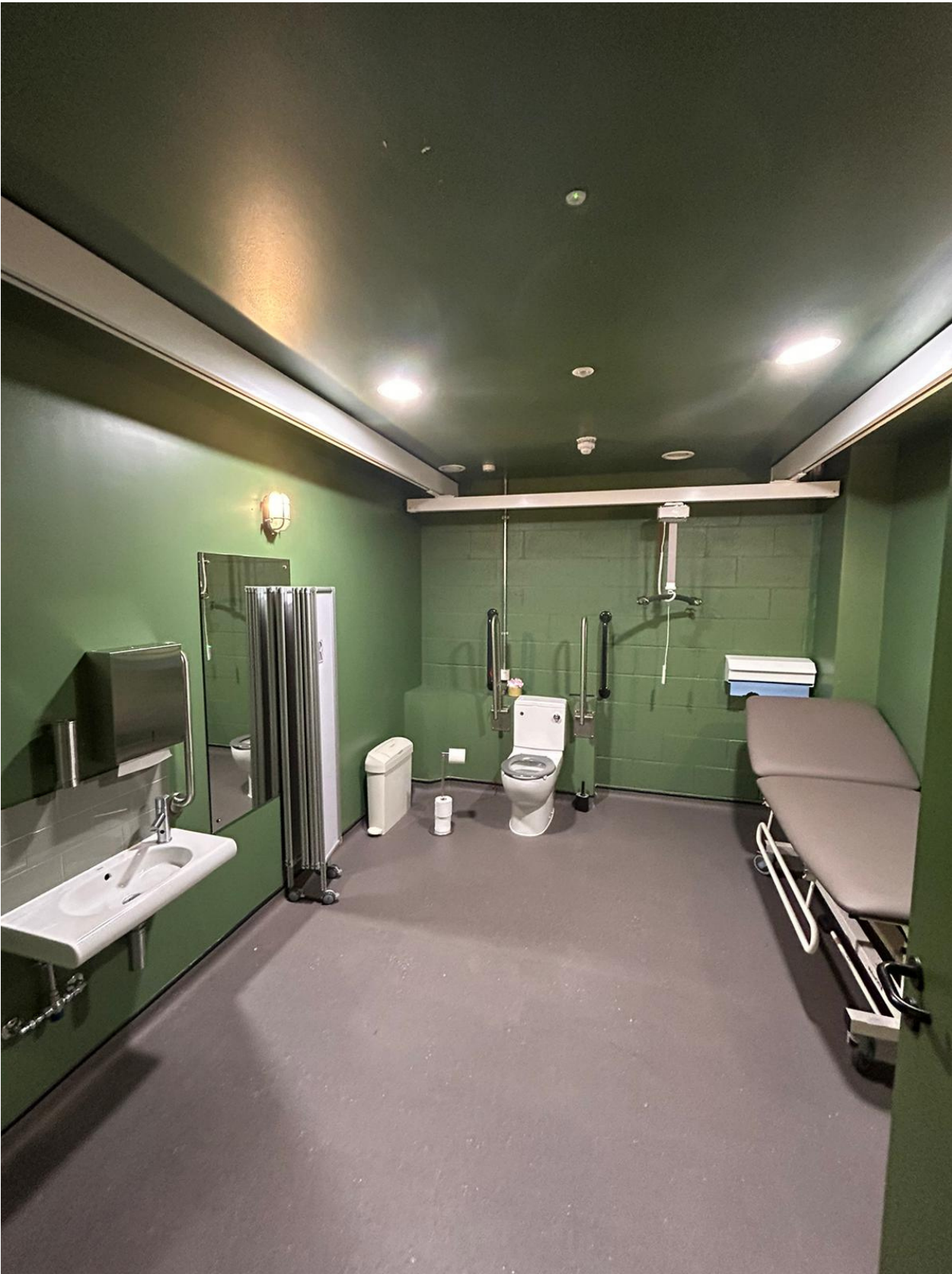
Disabled toilet changing space (Adult changing surface, hoist, privacy screen, support rails, emergency cord)
