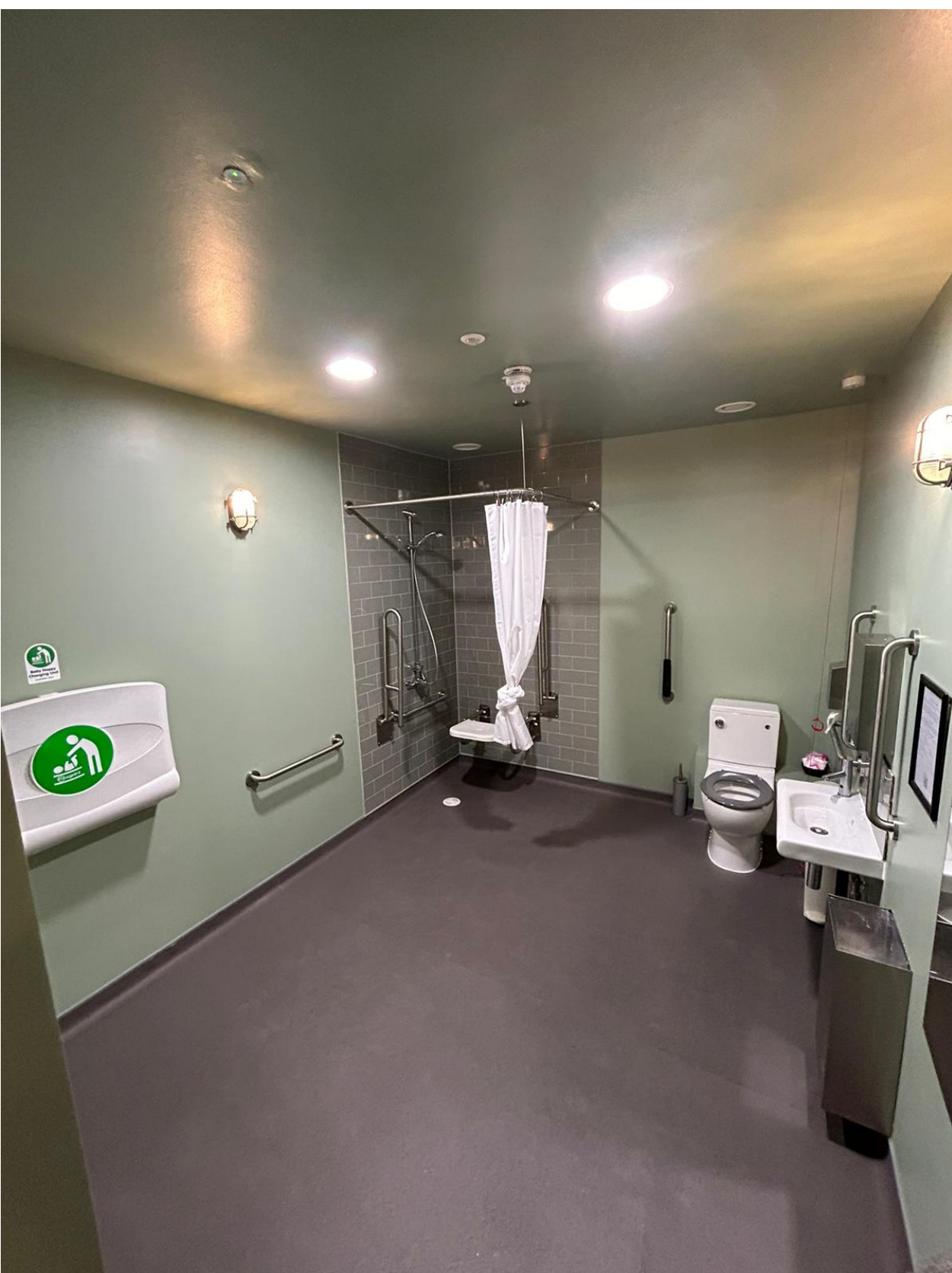
Disabled toilet and baby changing (Baby changing, shower, support rails, emergency cord)
