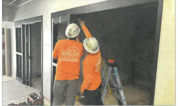
Perfection Glass installing sliding doors at Area B.2 Pre Post Surgery Rooms.
