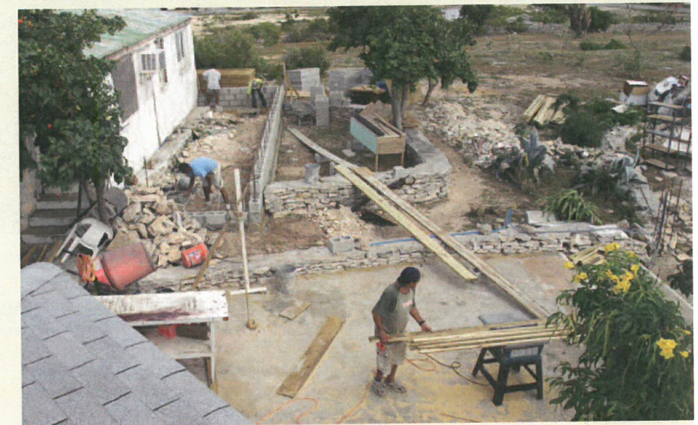
We were forced to suspend operations in the Turks and Caicos Islands from September-December 2008 due to damage from Hurricane Ike. In February 2009, we re-opened our center after extensive renovations to welcome 31 enthusiastic students.
