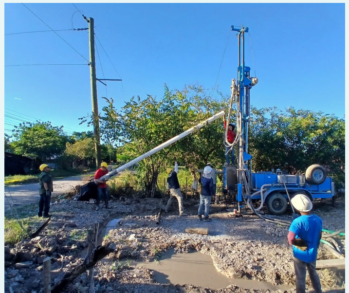
Living Water staff work hard to reach an underground aquifer at 42 meters. After testing and treating the water, they install a new hand pump.
