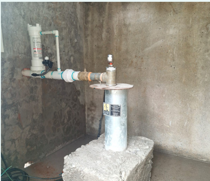
This piped water supply is insufficient and contaminated. Yet with no other options, residents are forced to use it.
