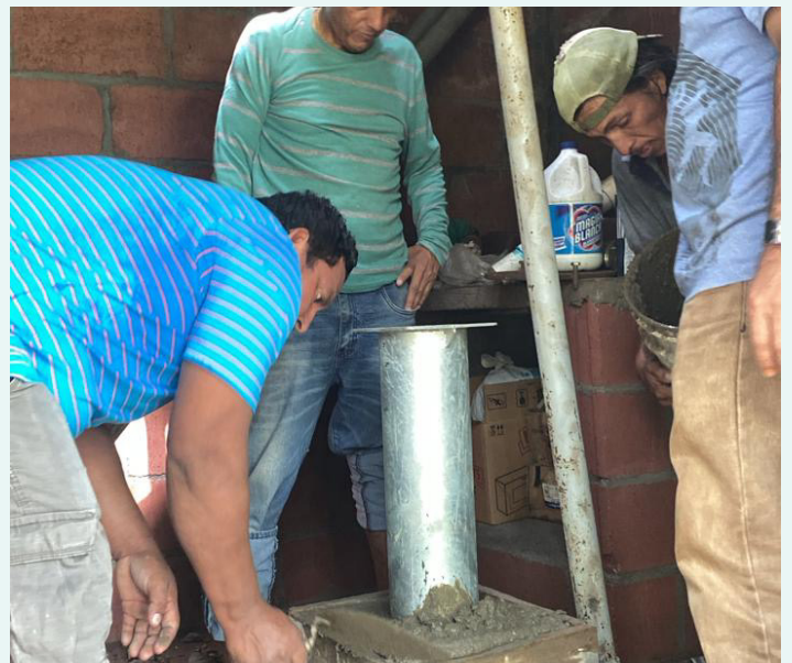
Reaching an underground aquifer at 90 meters, the team proceeds with safety checks and treatment before finalizing the project with a new piping distribution system.
