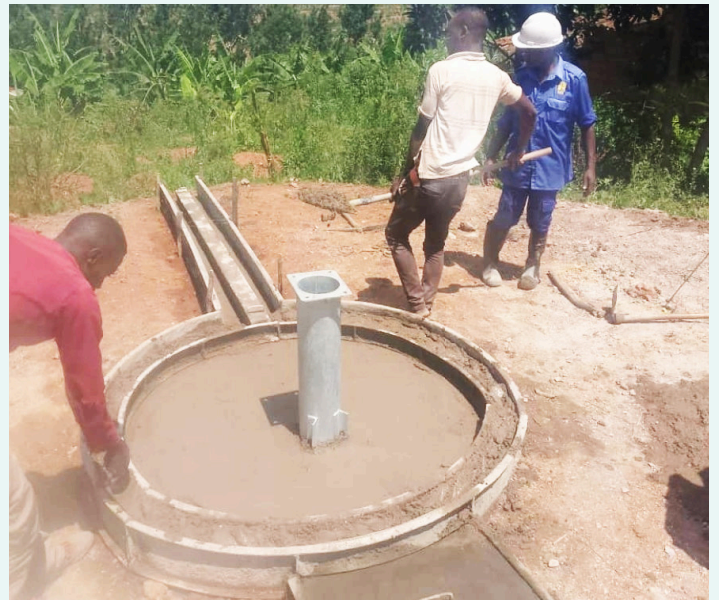
Reaching an underground aquifer at 70 meters, the team proceeds with safety checks and treatment before finalizing the project with a hand pump installation.
