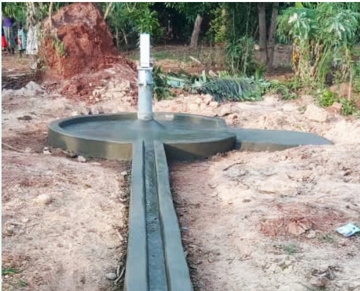
The new hand pump is complete! Residents now have reliable access to safe water.
