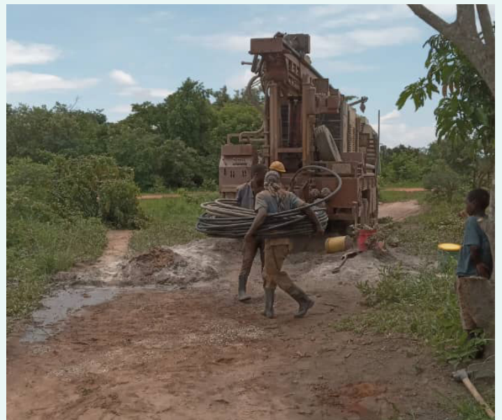
Reaching an underground aquifer at 56 meters, the team proceeds with safety checks and treatment before finalizing the project with a hand pump installation.
