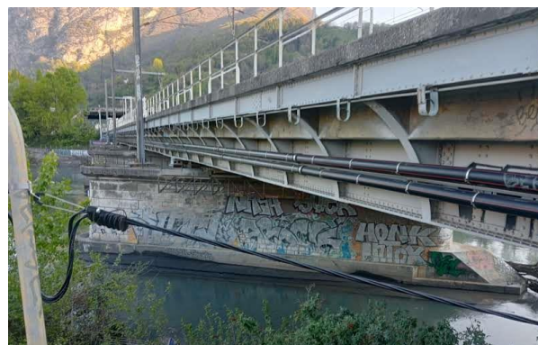
Figure 1: The railroad bridge monitored. The external metal girder on which the sensors are installed is visible.
