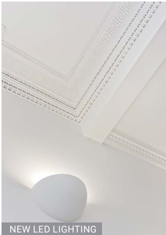
NEW LED LIGHTING
