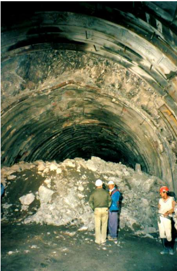
Figure 24: Large displacements in the top heading of the headrace tunnel of the Nathpa Jhakri Hydroelectric project. These displacements are the result of deteriorating rock mass quality when tunnelling through a fault zone.
