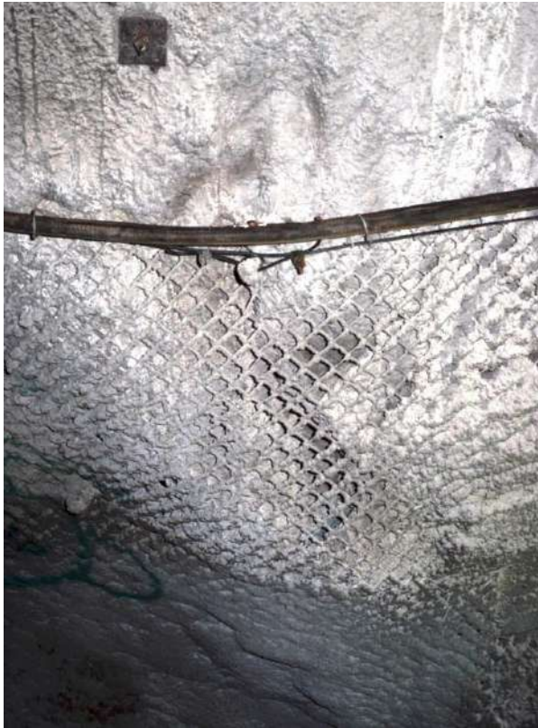
Figure 7: Chainlink mesh, while very strong and flexible, is not ideal for shotcrete application because it is difficult for the shotcrete to penetrate the mesh.
