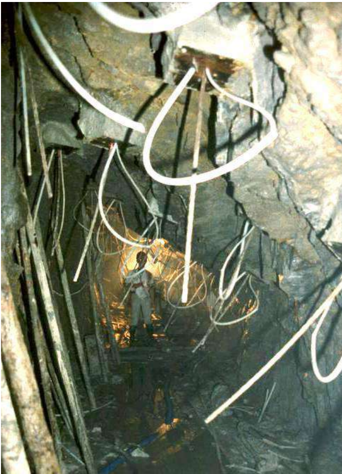
Figure 14: Untensioned grouted cables installed from the longitudinal working galleries to pre-reinforce the rock mass above the power cavern roof.
