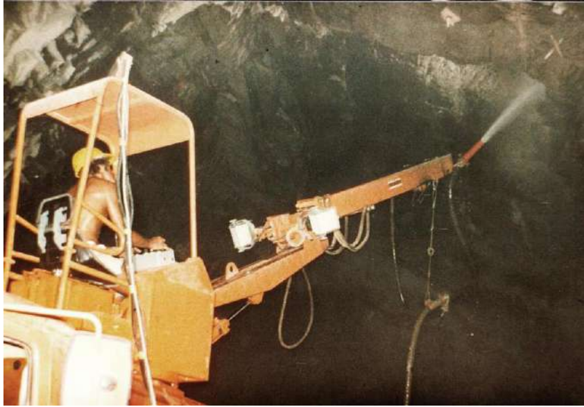
Figure 9: A truck mounted shotcrete robot being used in a large civil engineering tunnel. Note that the distance between the nozzle and the rock surface is approximately one metre.
