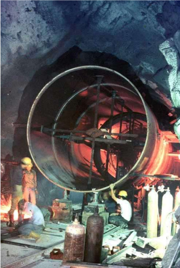
Figure 13: Installation of steel lining in a pressure tunnel in a hydroelectric project.
