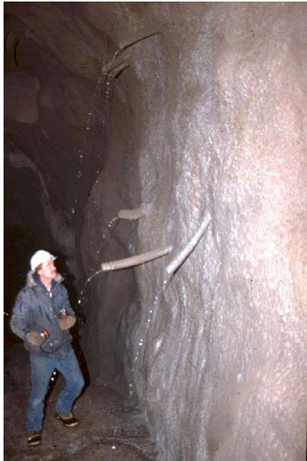
Figure 12: Plastic pipes used to provide drainage for a shotcrete layer applied to a rock mass with water-bearing joints.
