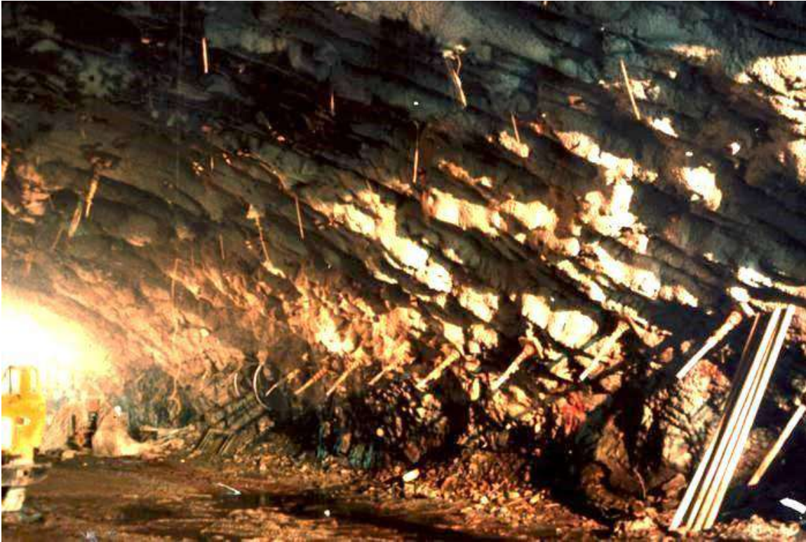
Figure 18: Blast damage in the first section of the cavern arch to be excavated.
