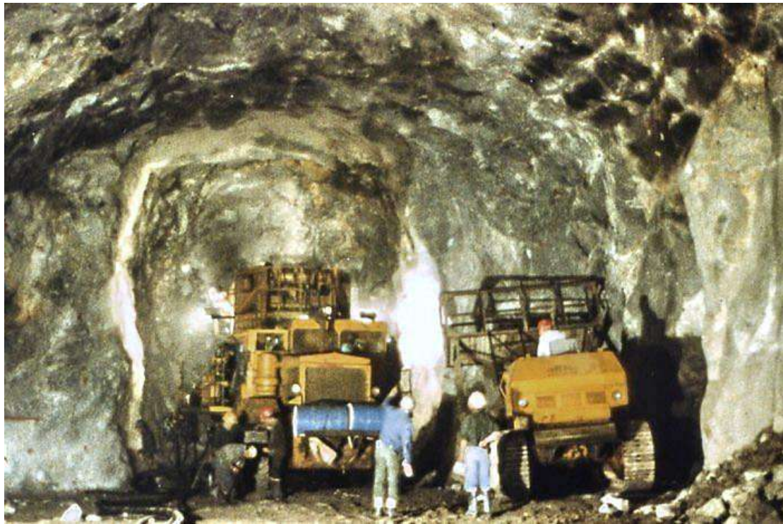
Figure 4: A 6 m wide heading driven ahead of the tunnel face to permit pre-reinforcement of potentially unstable wedges in the roof. The seven-boom jumbo is seen working in the heading.
