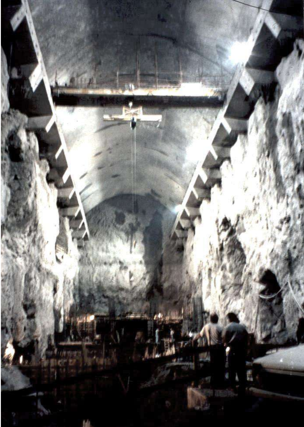
Figure 29: Crane beams rockbolted to the walls of the power cavern of the Thissavros hydroelectric project in Greece. These rails provided support for the temporary construction crane shown in the photograph. The stubs projecting from the bottom of the beams were later attached to concrete columns that provided support for the main crane.
