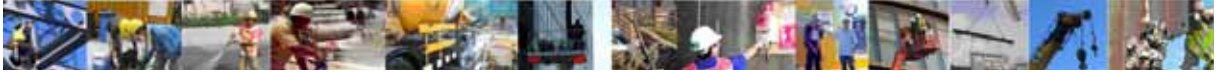
Workers at the bottom of excavation (with temporary walkway and latrine facilities)
