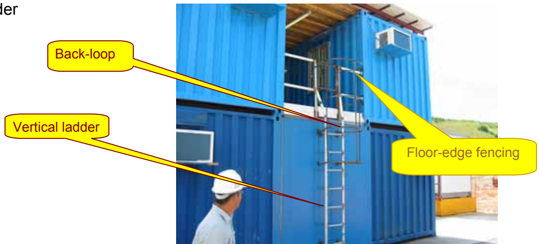
Typical fixed inclined ladder
