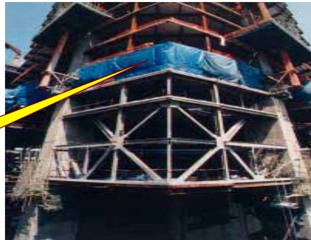
Fenced external frame
