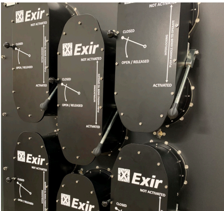
1. Example of Patch Panel in normal mode.
